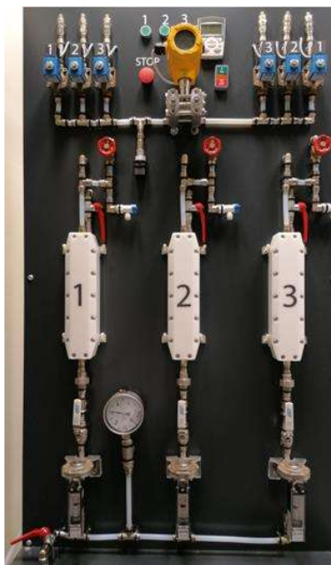
Fig. 1. The photo of experimental pilot-scale crossflow UF membrane filtration system.
